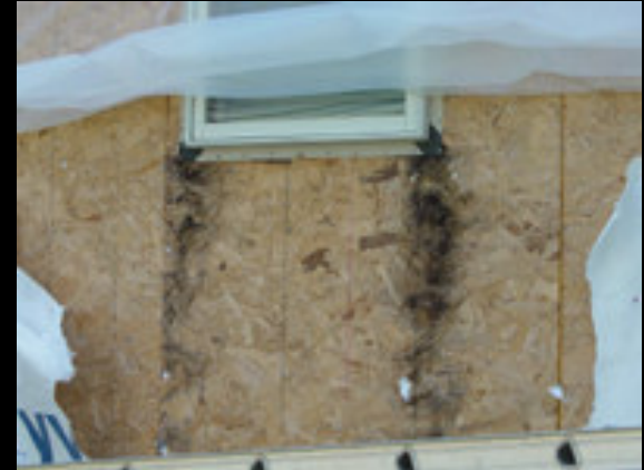
Fungal contamination and rot
