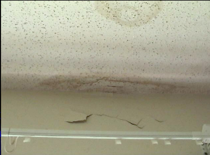
Ceiling and drywall damage
